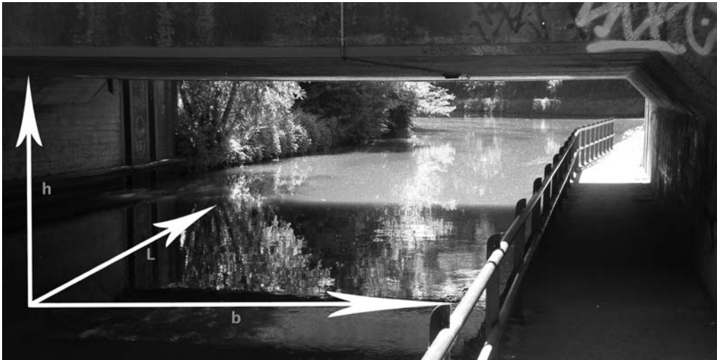
Photo 4. Length (L), height (h) and width (b) of a culvert. Photograph: M. Boonman
